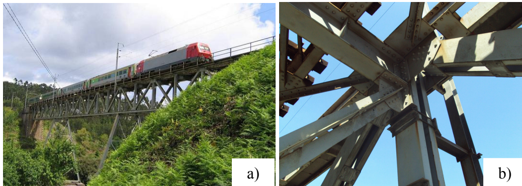
Figure 1: Riveted railway Trezói bridge: a) overview of the bridge; b) node under investigation.
