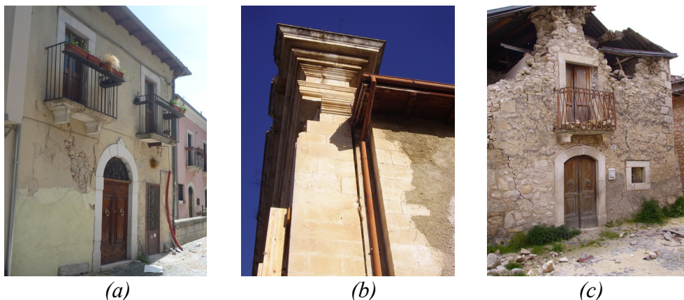
Figure 8. Main global collapse mechanisms: (a) in-plane, shear failures due to diagonal shear cracks in the masonry piers; (b) out-of-plane overturning; (c) diagonal wedge and horizontal bending.
