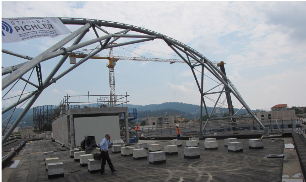
Figure 3: the pre-assembly phase of the steel tubular system to support the structural membrane (Courtesy of Studio Ossola)
